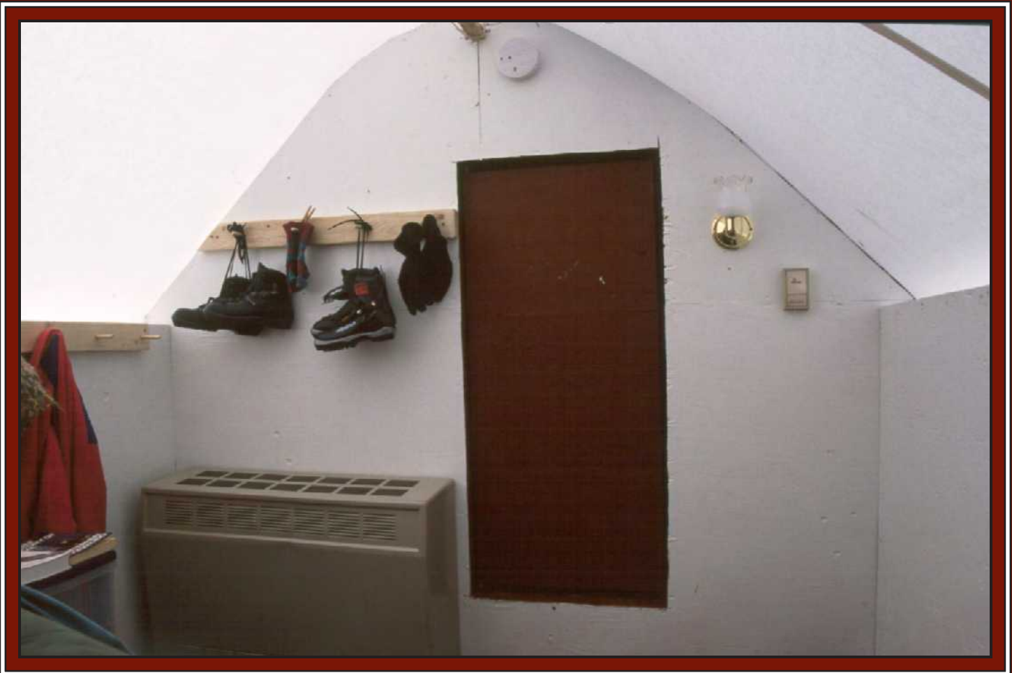
Each private sleeping hut has its' own heater, thermostat, and solar powered electric lights, plus lots of hooks and clothes lines for drying gear
